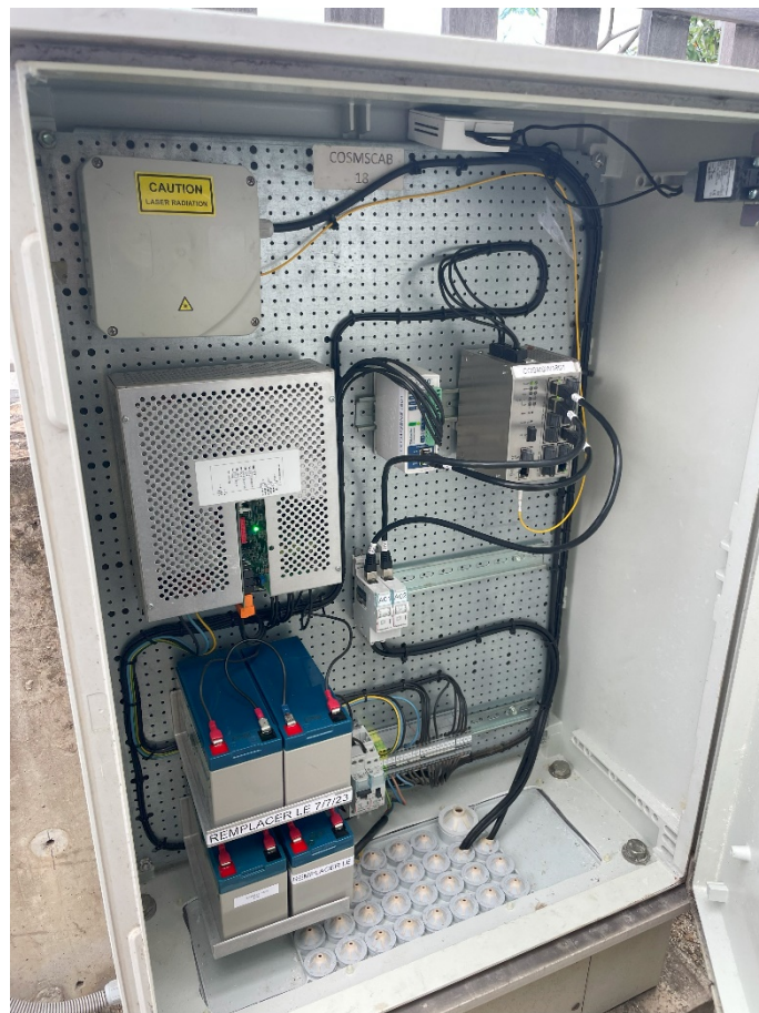
Figure 39 : Raccordements internes au coffret
